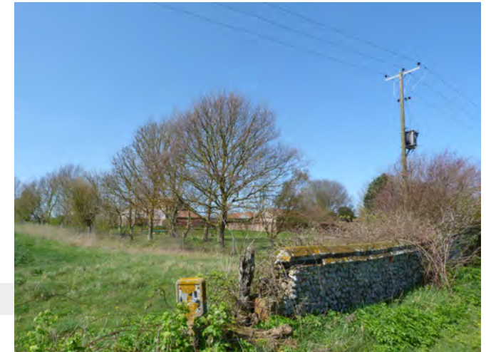
Damaged wall at south-east corner of the Conservation Area [NB: not currently in Conservation Area but would be if boundary was amended]
