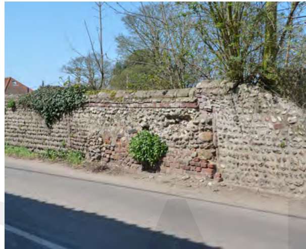
Damage to boundary wall on The Street, with vegetation growth present
