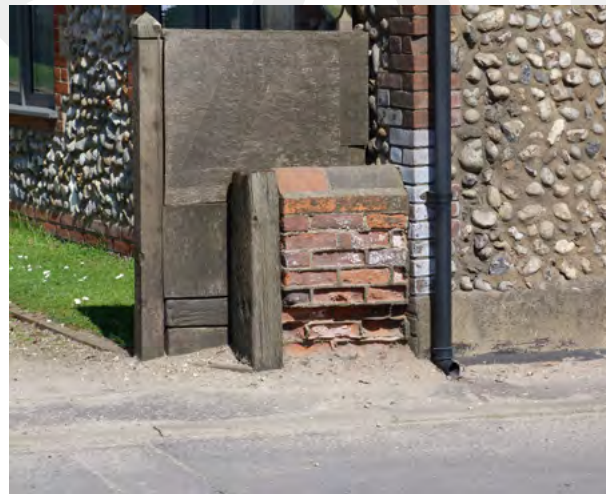
Worn bricks, caused by water splashing up from the road from passing vehicles
